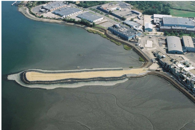
31. Full aerial view of Causeway at completion of sand application, (photo courtesy of R. F. Weston).
