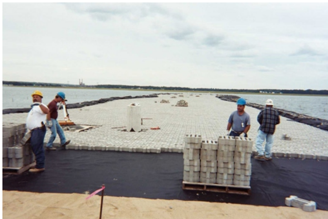
23. Deployment of articulating concrete block over woven geotextile, all deployment was performed by hand. Note concrete light pole base in immediate background.
