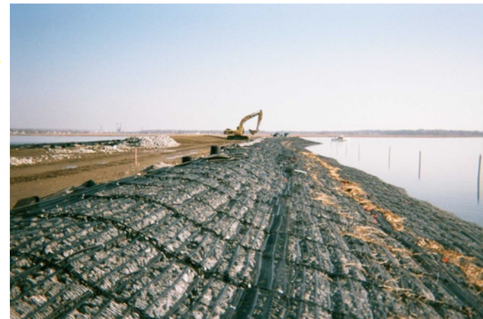
16. Completed area of marine mattress on east side of causeway. Note red flagging indicating QA inspection identified deficiencies.
