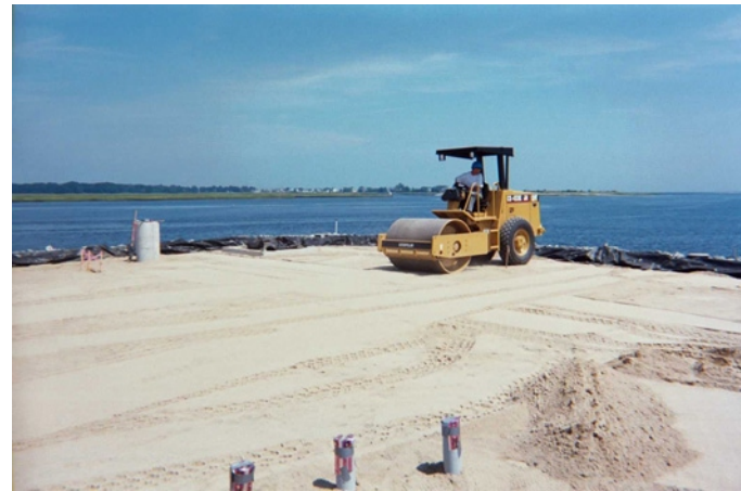
22. Application of bedding sand and compaction prior to articulating concrete block deployment.
