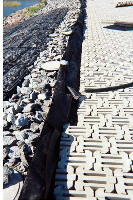
26. Final detailing of articulating concrete block along rip rap apron. Geotextile layer intended to retain vegetative soil from migration into rip rap stone.
