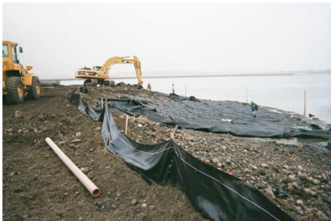
11. Deployment of lower cover system marine mattresses over woven geotextile. Elevation 6.0 MSL is at silt fence line.
