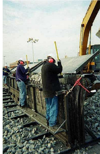
6. Detail of aggregate filling operations for marine mattress. Note tamping of stone into mattress baffles.
