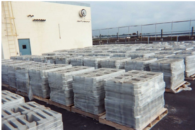
21. Pallets of articulating concrete block staged near Building No. 4 inside south guard post.
