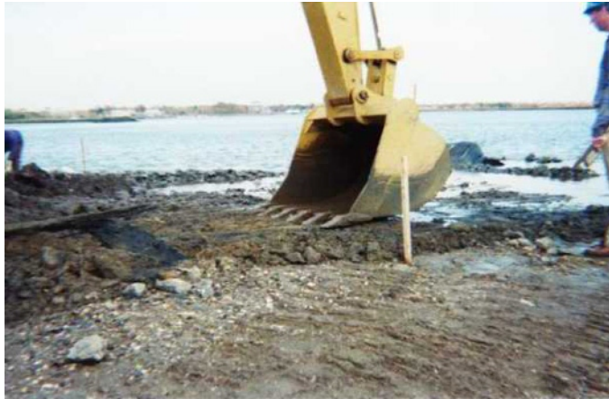
1. Subgrade soil, 1-foot cut to accommodate lower cover system marine mattresses placement.
