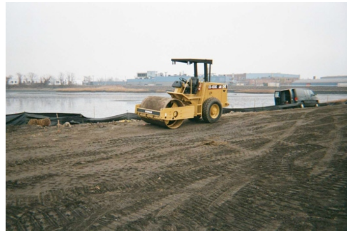
2. Compaction of acceptable subgrade fill in upper cover area (static load only).
