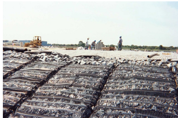
24. Transition from marine mattress to rip rap apron to upper cover system looking to the south west at approximate baseline station 5+50.
