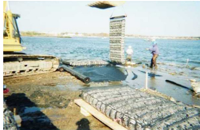
4. Marine mattress deployment at low tide (looking north towards Housatonic River channel).
