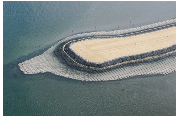
32. Aerial view of Causeway tip post bedding sand application. Note grayish color of marine mattresses indicating algae growth, (photo courtesy of R. F. Weston).
