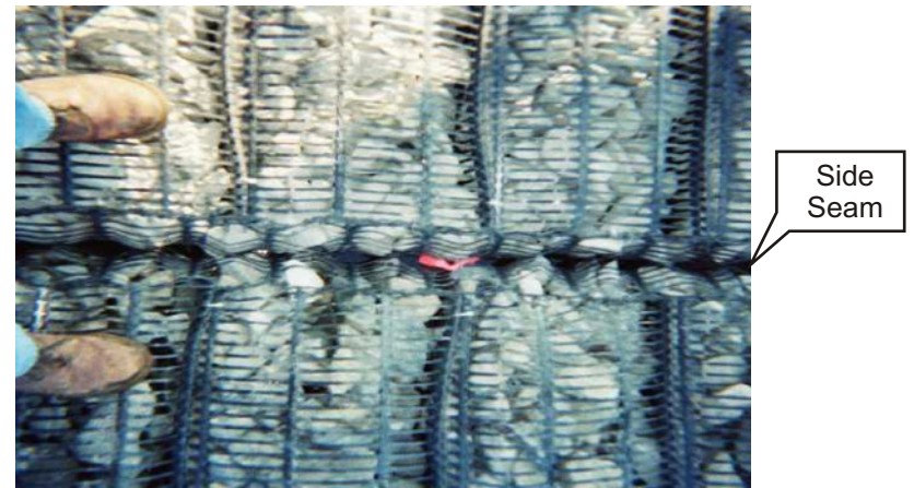
14. Deployed marine mattress side seam gap. Note individual baffle pillows within mattress units.
