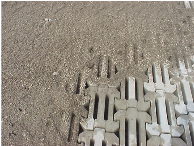
29. Filling of articulating concrete block with interstitial gravel fill (photo courtesy of R. F. Weston).
