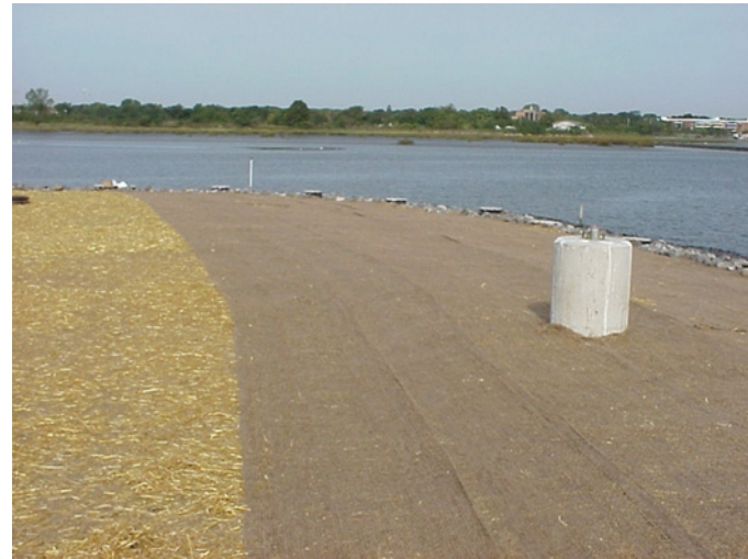
30. Looking north along Causeway with final grading, jute mat application and straw mulch, (photo courtesy of R. F. Weston).
