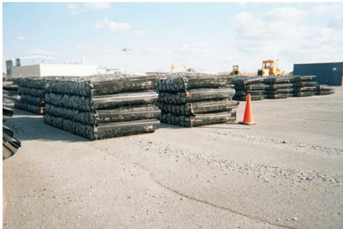
9. Marine mattresses staged in South Parking Lot after fabrication. Note QC flagging on individual units.
