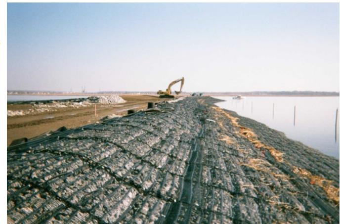
16. Completed area of marine mattress on east side of causeway. Note red flagging indicating QA inspection identified deficiencies.
