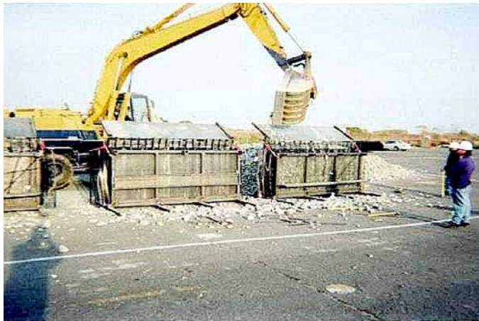
5. Filling factory fabricated marine mattresses with crushed D50 = 3-inch aggregate in South Parking Lot SAEP.
