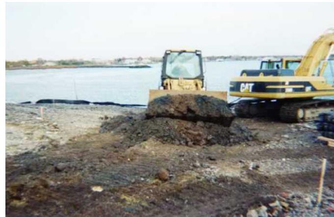
8. Relocating subgrade spoil excavation from lower cover system for scarification and drying.
