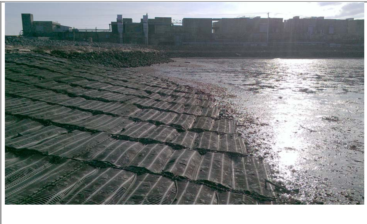
Photograph 28: Additional west slope view
