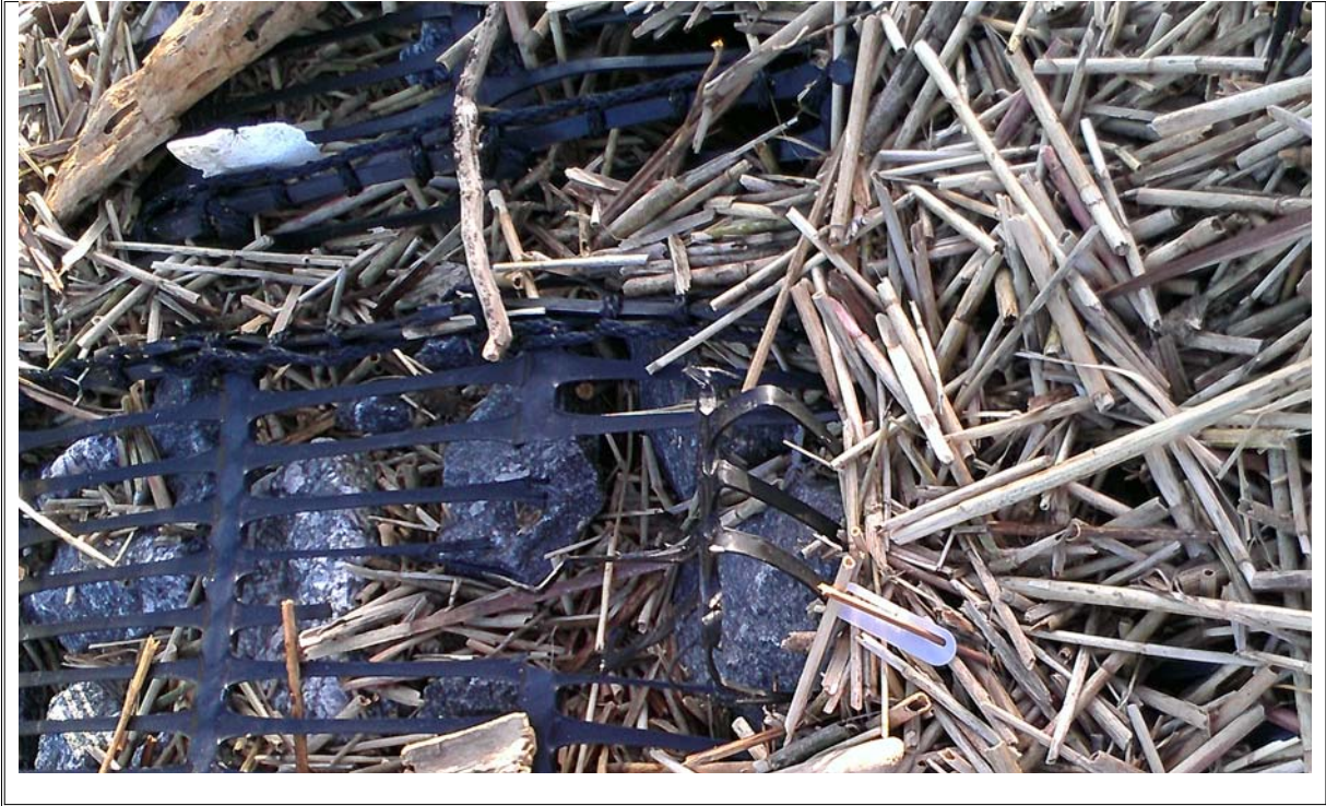
Photograph 23: Marine mat at eastern end of causeway showing minor tear
