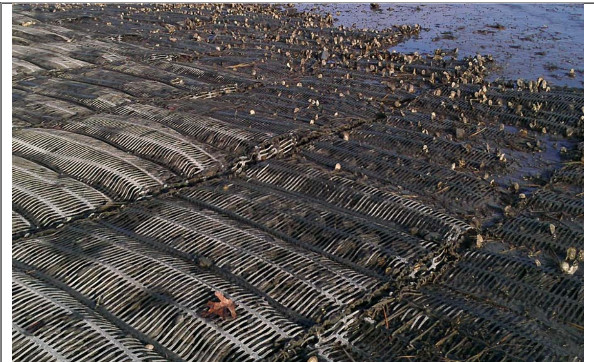
Photograph 24: Marine mat at eastern end of causeway showing minor differential settlement
