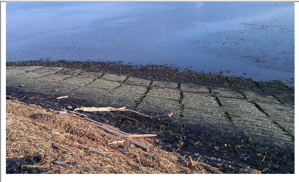
Photograph 22: Marine mat at eastern end of causeway showing minor differential settlement
