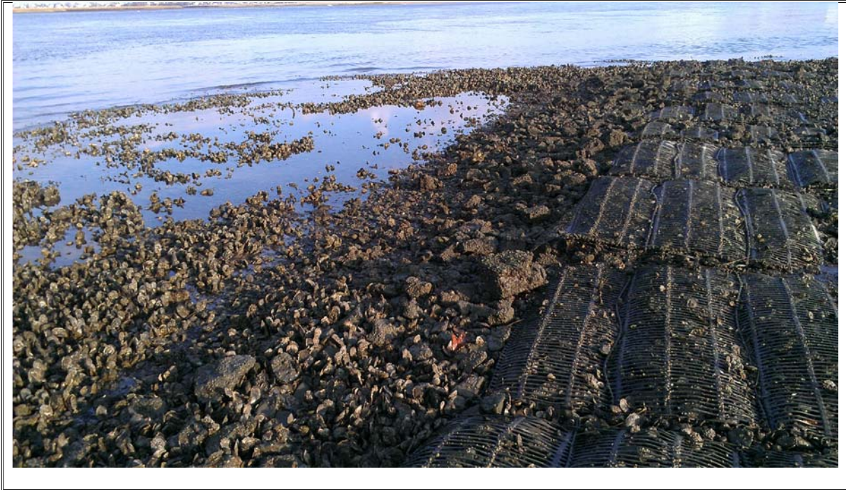
Photograph 13: Eastern tip of causeway showing cobble and shellfish accretion on marine mat
