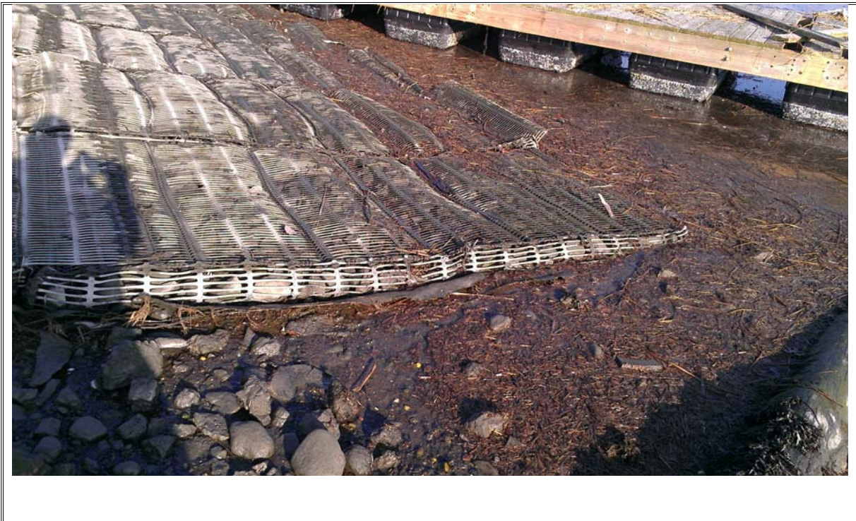
Photograph 32: View of eastern face of causeway showing mat/riprap transition, view to southwest
