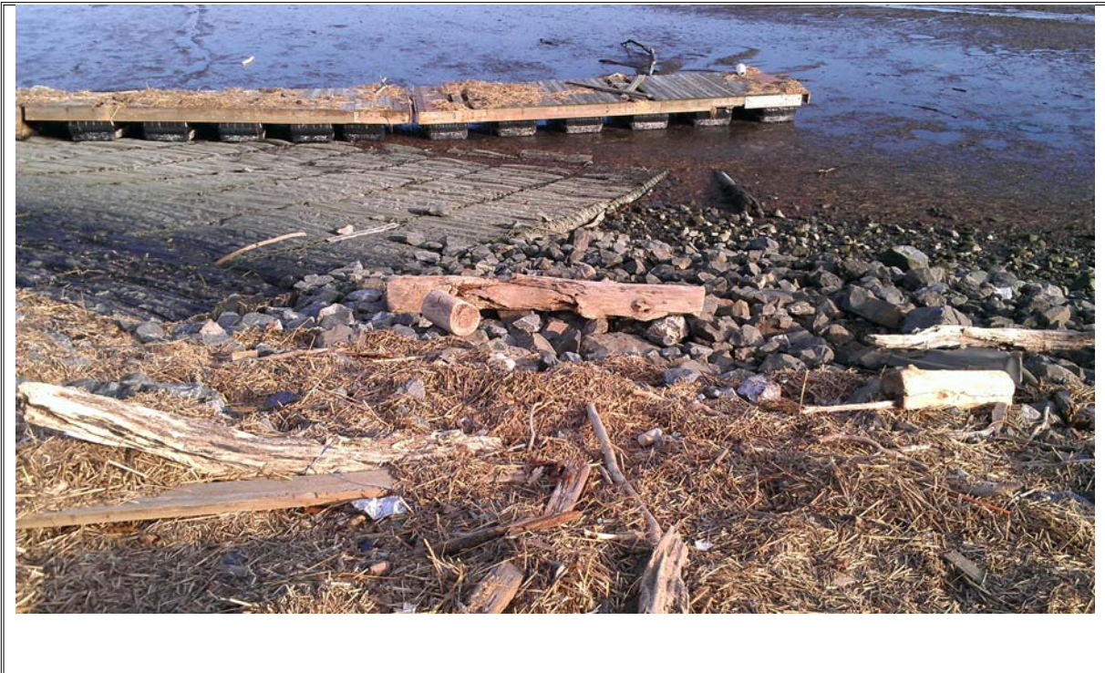
Photograph 10: View of southwest slope of causeway. Driftwood stump and floating dock structure deposited during passage of Hurricane Sandy on 29 October 2012
