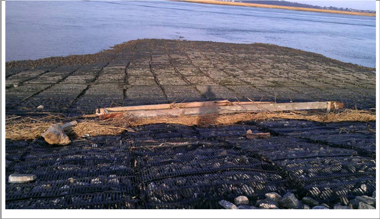
Photograph 19: Eastern tip of causeway showing general marine mat condition and storm debris
