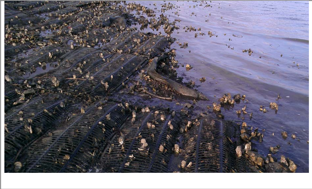
Photograph 18: Marine mat edge at northeast tip of causeway showing minor woven geotextile base exposure, second view
