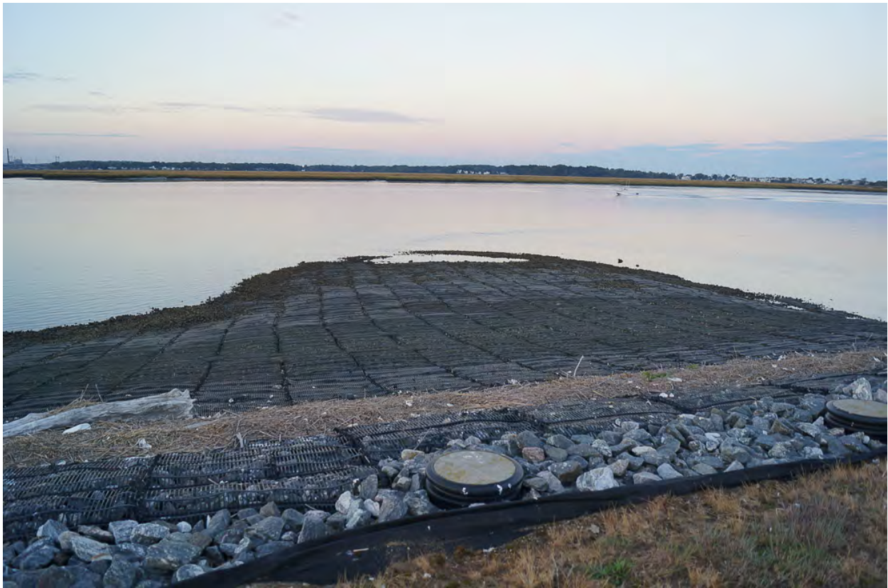
Photo 17. North Causeway looking north across Housatonic River towards Nells Island, near low-tide. Note shallow slope of marine mattress erosion control cover system extending to subtidal. October 6, 2017.
