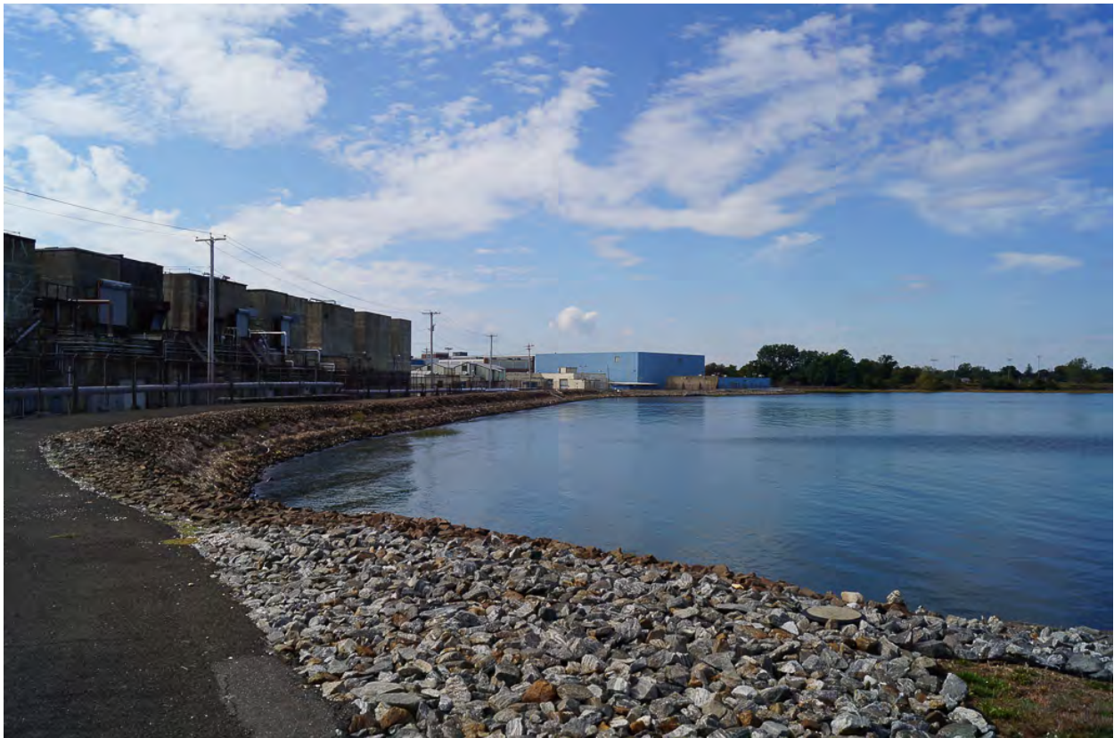
Photo 5. Head of Causeway looking west across west tide flat, dike and revetment, mid-tide. October 6, 2017.
